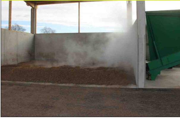
In the dryingbox we use the excess energy of the pyrolysis-process
