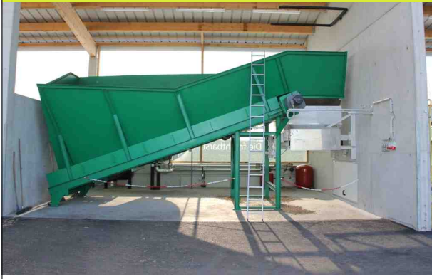
The loading is large enough for the daily requirement of fuel
